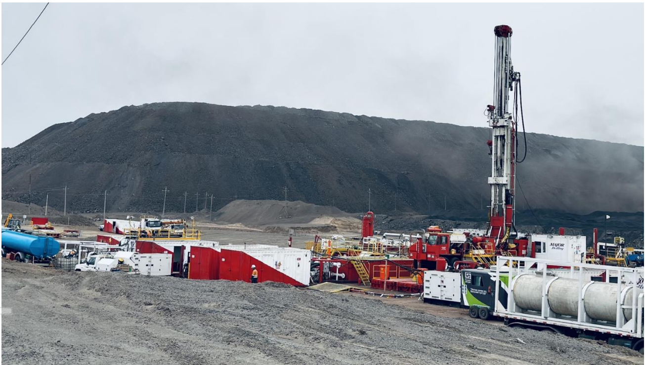
Figure 1 – Major Drilling Rig on location for the Lucky Fox - 2 pilot production well
